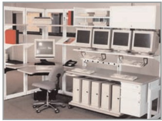
Network Storage Rooms
